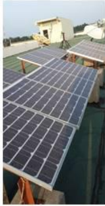
Solar Panels (1.5 kW)
