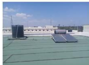
SOLAR WATER HEATER
